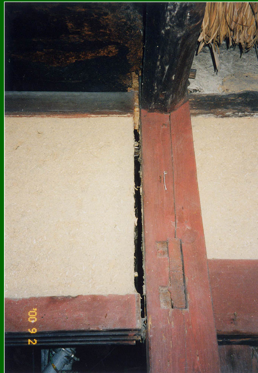
垂壁と柱の剥離( 1/30\text{rad.} )
